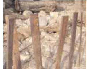
Failed barrier fence and rip-rap
